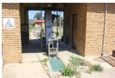
Inlet Structure with mechanical screen
