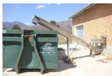
Dry sludge conveyor system (Huber)
