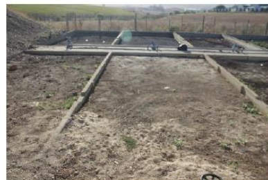
Sludge drying beds
