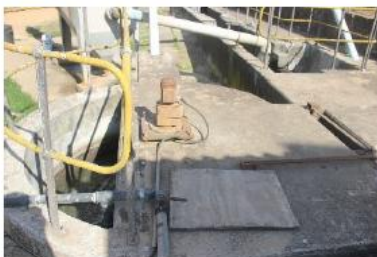
Inlet structure: Two vortex degritters
