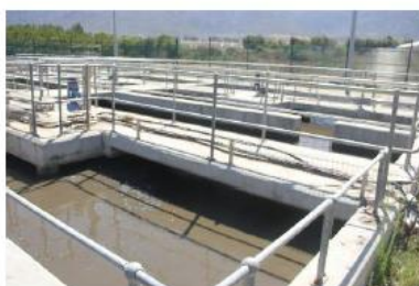
Reactor: Anaerobic Zone
