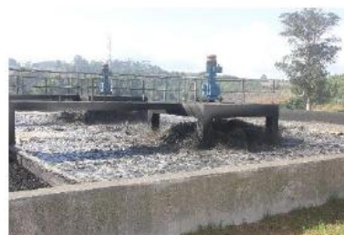
Reactor: Aeration zone
