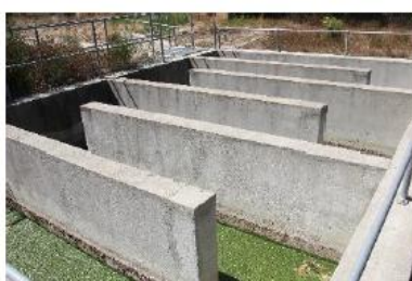
Chlorine contact channel
