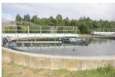
Secondary Settling Tank No.5
