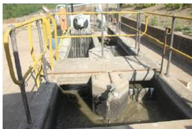
Inlet structure with mechanical screens
