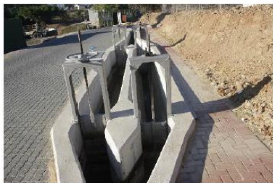
Inlet works with two grit channels
