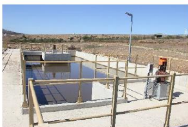
Reactor: Anaerobic zone with two mixers
