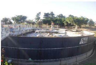
Sequencing Batch Reactor, with floating aerators
