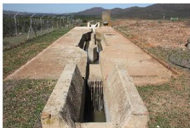
Inlet Structure with hand raked screen
